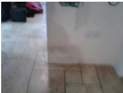
Figure 4.11 Area of remaining damp in Grove Cottage
