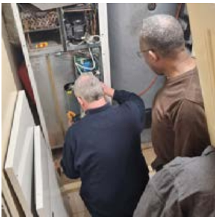
Figure 8.7 Princedale Road: maintenance of MVHR fan within the Genvex combined unit (MVHR hot water cylinder and air source heat pump)
