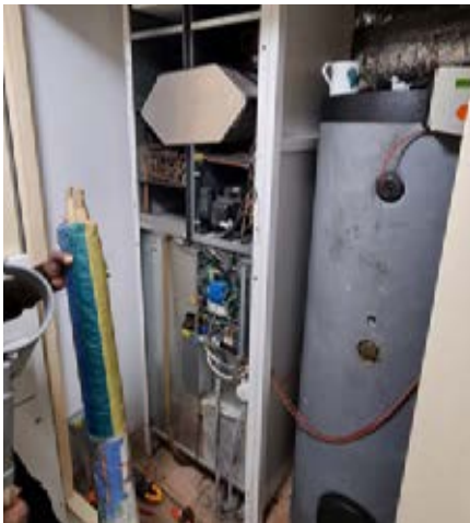
Figure 8.3 Princedale Road: GenvexCombi providing hot water and fresh air supply throughout the house; set behind acoustic doors
