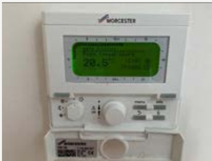
Figure CS6.6 Worcester heating controls in hallway
