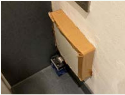
Figure CS6.5 Low level extract unit in WC
