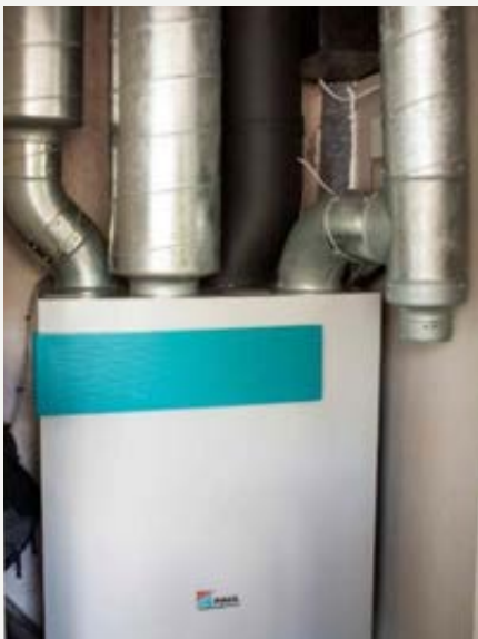
Figure CS1.6 MVHR unit and related ducts
