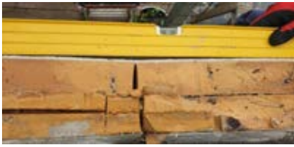
Figure 4.3 Blaise Castle: phenolic insulation board has bowed
