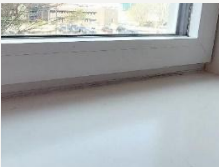
Figure CS9.5 Mould to the window seal in upstairs bedroom
