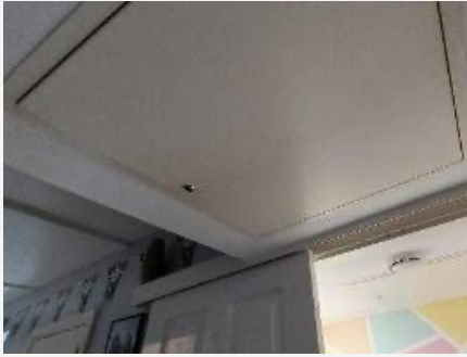
Figure CS9.4 Access panels to MVHR duct distribution in the hall and WC
