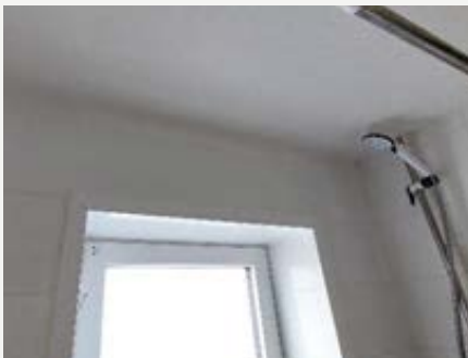
Figure CS9.6 Evidence of mould to the ceiling in the upstairs bathroom
