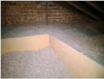
Figure CS1.5 Cellulose roof insulation covering the MVHR ducts
