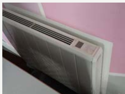
Figure CS9.3 The only radiator in the maisonette with on/off switch only
