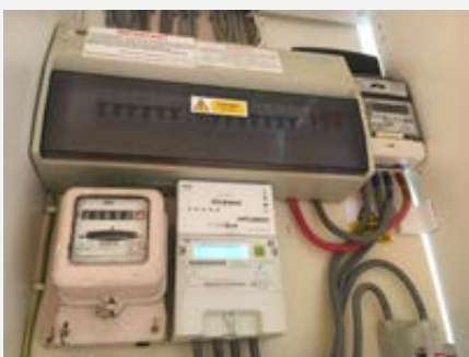
Figure CS7.6 Electric consumer unit and meters; the old meter had not been removed
