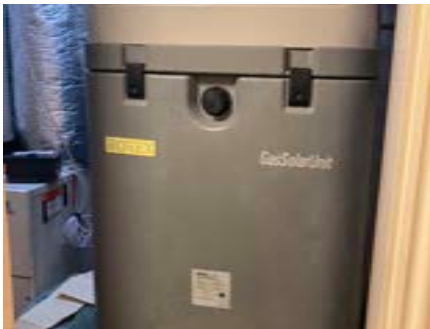
Figure 7.4 Hawthorn Road Rotex Gas Solar Combi Unit provides heating and DHW
