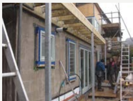
Figure CS1.2 Original Finlock gutter; gutter being cut off; eaves extended with insulation between rafters; EWI interface with roof insulation in new soffit zone
