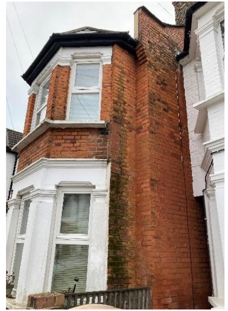
Figure CS2.6 Front elevation showing impact of leaky gutter on brickwork
