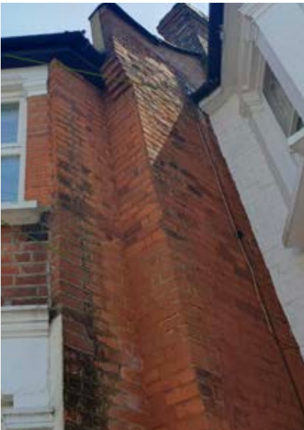
Figure CS2.7 Freeze-thaw damage at high level as a result of faulty rainwater goods, primarily exacerbated by inappropriate cement pointing. Cryptoflorescence visible. The IWI may be increasing the risk, but to a lesser degree than the cement
