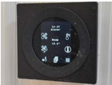
Figure 7.6 Princedale Road GenvexCombi unit controls with easy icons but quite complex to operate
