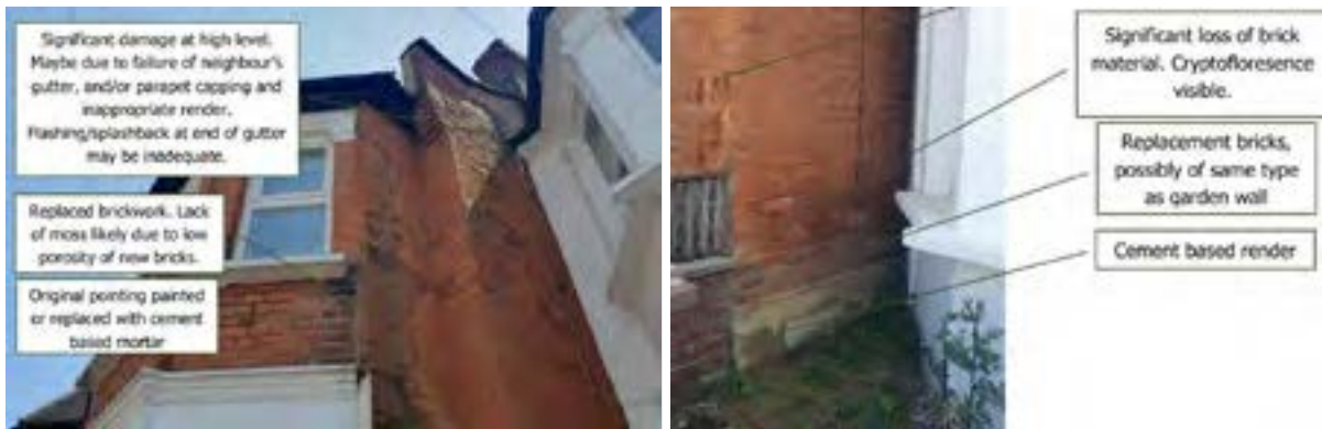
Figure 4 Damage near the gutters (left) and above the ground floor (right) on the west wall
