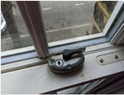
Figure CS8.5 Sash window seal missing to the left of the window catch, contributing to the increased permeability.
