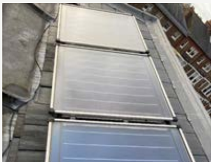
Figure CS6.7 Solar thermal panels
