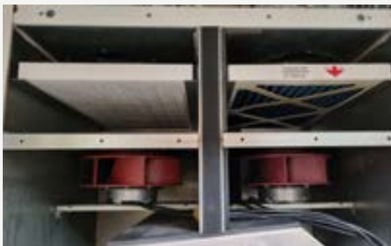
Figure CS7.8 MVHR fan and filters in the Genvex unit
