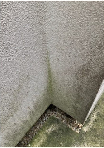
Figure CS2.4 Light moss and weathering on external wall insulation render
