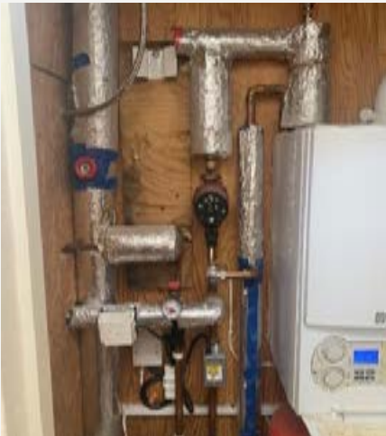
Figure CS3.2 Insulated pipes throughout the property
