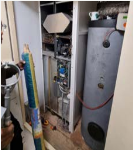
Figure CS7.4 Utility cupboard with MVHR hot water and mini air source heat pump next to complimentary hot water cylinder
