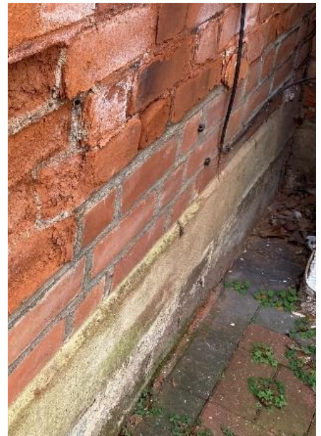
Figure CS2.9 Salt crystallisation damage near to ground level as a result of rising damp (likely linked to the floor treatment), primarily exacerbated by inappropriate use of cement (and possibly impermeable paint)
