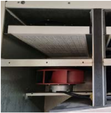
Figure 8.2 Princedale Road: MVHR fan and filters, left hand fan has been replaced after functioning for 11 years
