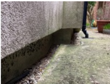
Figure 5.7 Slight staining of the EWI render
