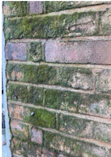
Figure CS2.8 Moss growing on brickwork due to excessive moisture exposure
