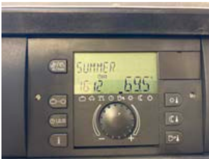
Figure 7.5 Hawthorn Road Rotex Gas Solar Combi Unit controls were more complex to operate than expected and lead to difficulty in operating the system for the tenant
