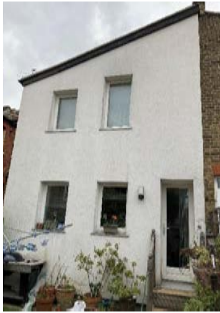
Figure CS2.5 Rear elevation external wall insulation in good condition with very few hairline cracks in render
