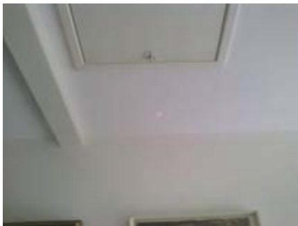
Figure 4.4 Ceiling examined by thermal imaging
