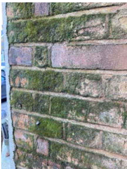
Figure 8.1 Hawthorn Road: moss on brick wall by leaky gutter
