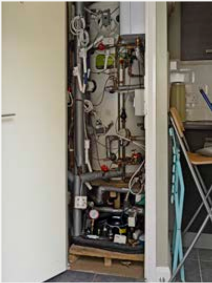
Figure CS8.4 Utility cupboard with conflicting MEP installation
