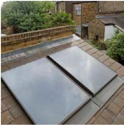
Figure 8.6 Princedale Road: solar thermal panel on the roof
