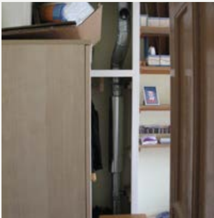
Figure CS10.2 Ventilation duct concealed in wardrobes
