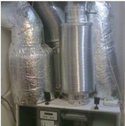
Figure CS2.3 MVHR unit with primary ducts insulated
