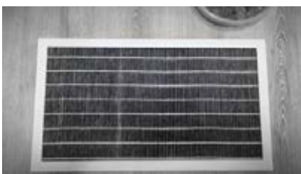
Figure 8.8 Princedale Road: MVHR filter clogged up with particles and pollution
