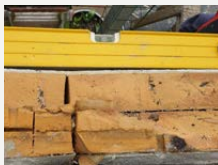
Figure CS1.3 Recent exposure of EWI (April 2023) above balcony section undergoing repairs
