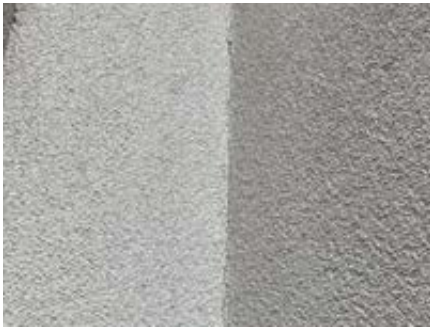
Figure 5.6 Minor hair line crack in external wall insulation (EWI) top render
